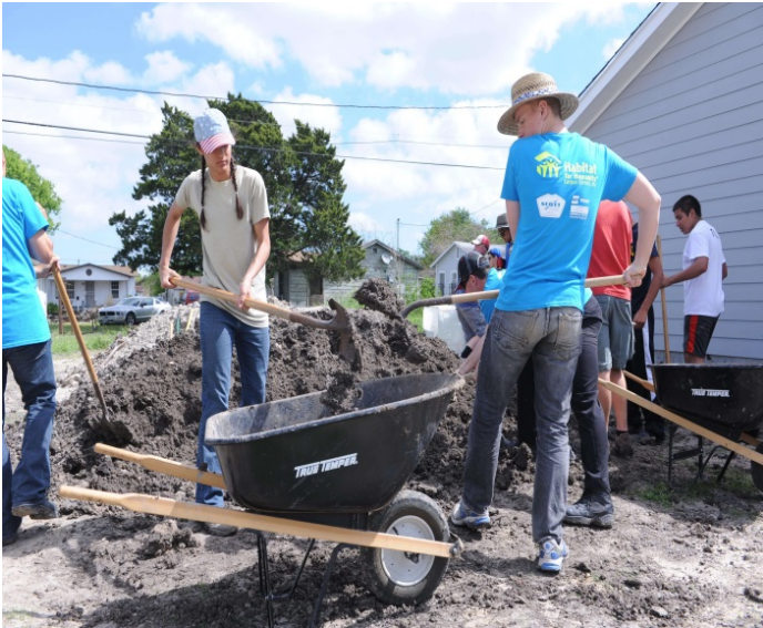
Then-Cadet 2nd Class Leah Gates (left) and then-Cadet 4th Class Luke Robinson shovel dirt into a wheelbarrow in Corpus Christi, Texas, March 22, 2017, during an Alternate Spring Break Program volunteer effort with Habitat for Humanity. (Air Force photo/John Van Winkle)
